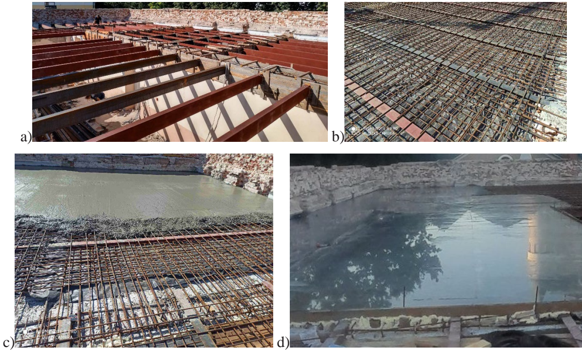
Fig. 1. Stages of resource-saving built-in composite steel-reinforced concrete floor construction: a) load-bearing steel beam layout; б) monolithic reinforced concrete slab working reinforcement installation; в) monolithic slab concreting process; г) general view of the slab immediately after concrete mix placement and compaction
