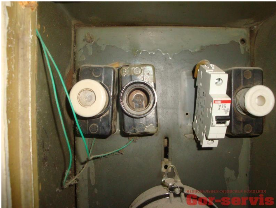
Figure 1.1 – Existing outdated equipment
