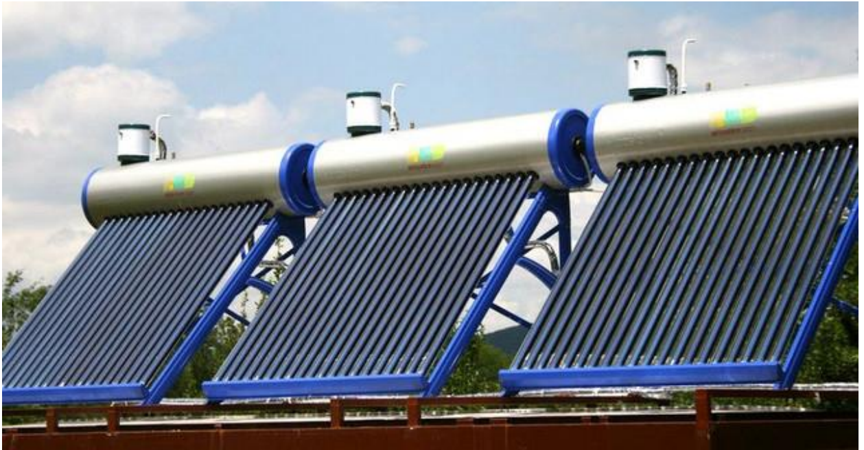
Figure 1.6 – Solar collectors for heating and hot water
