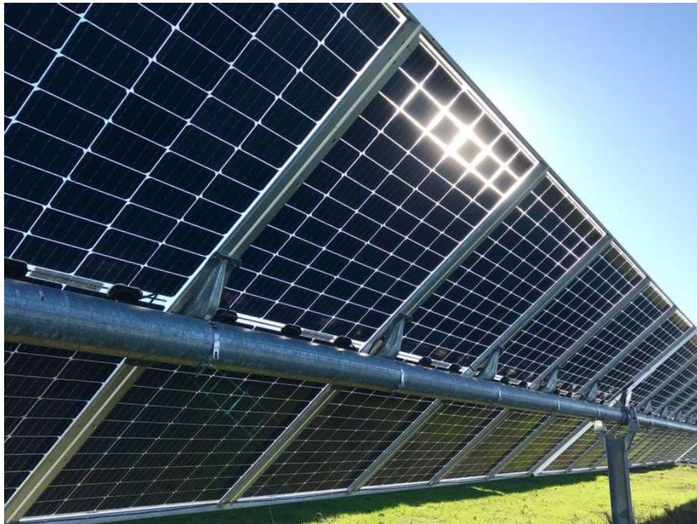
Figure 1.1 - Bifacial solar panels.
