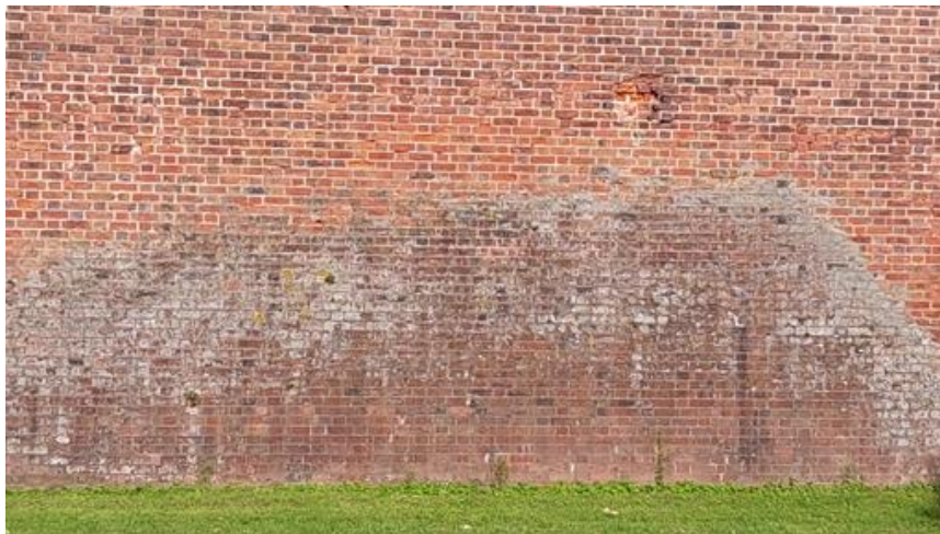
Fig. 10. Salinity at a considerable height of brickwork, 2025
