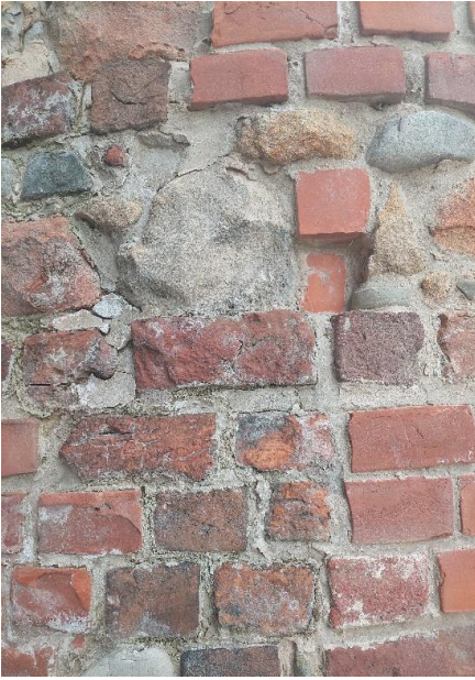
Fig. 4. Castle in Oświęcim. Peeling off ancient mortar (2024)
