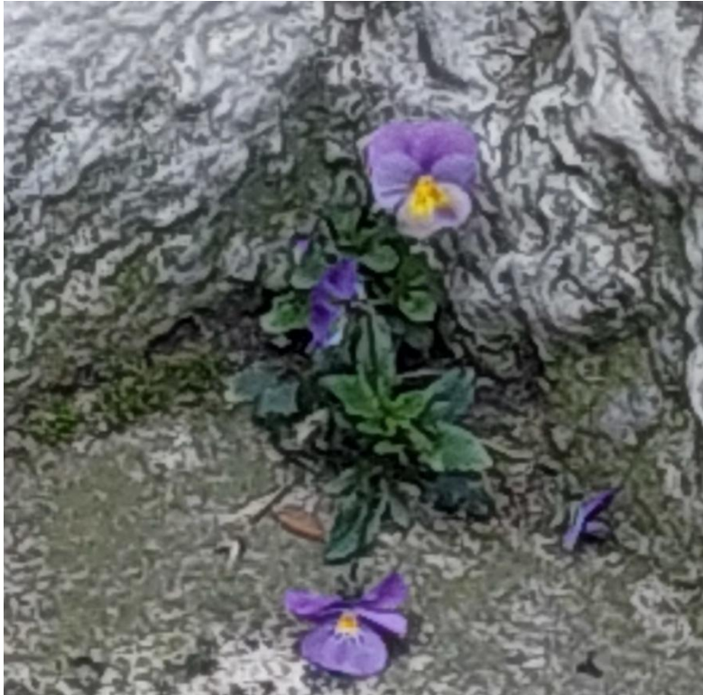
Fig. 2. Biological damage to the lower part of the walls.
