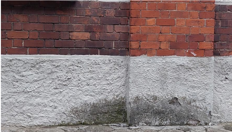
Fig. 2. Moisturizing and salinization of the wall.
