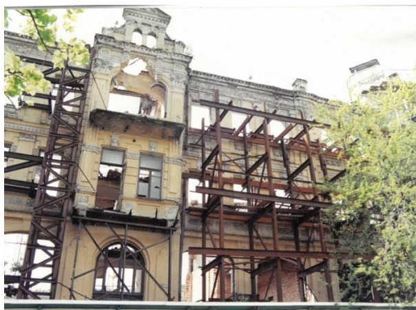
Fig. 7. Condition of the walls of a building in the Bessarabskyi quarter in Kyiv before the start of restoration (2001)
