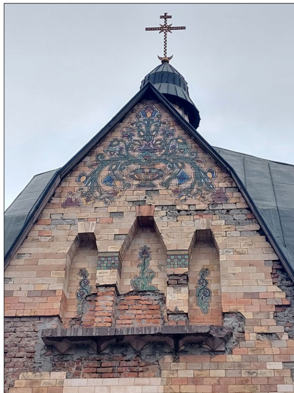
Fig. 7. Current condition of ceramic tile cladding on the eastern facade of the chapel; photo by Y. Ivashko, 2025
