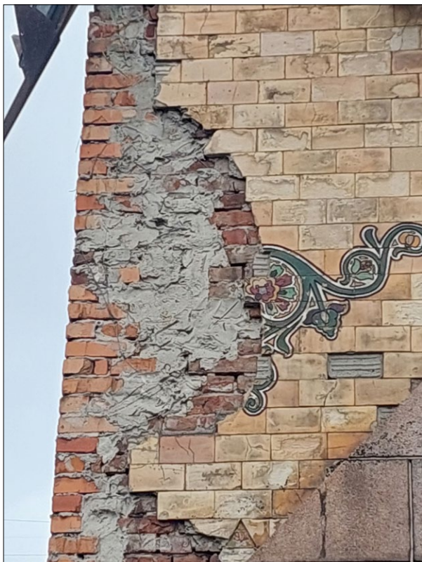
Fig. 6. Brickwork restored with modern bricks at the corner of the chapel; photo by Y. Ivashko, 2025
