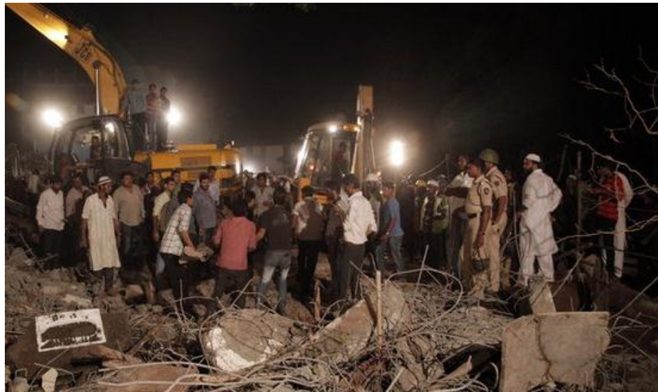
Fig. 3.2. Collapse of the house which was in process of construction, Mumbai, India, 2013
