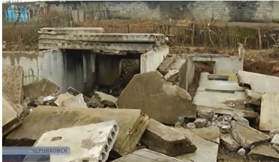
Fig. 3.1. Collapse of the unfinished building, Cherniakhovsk, Russia, 2015
