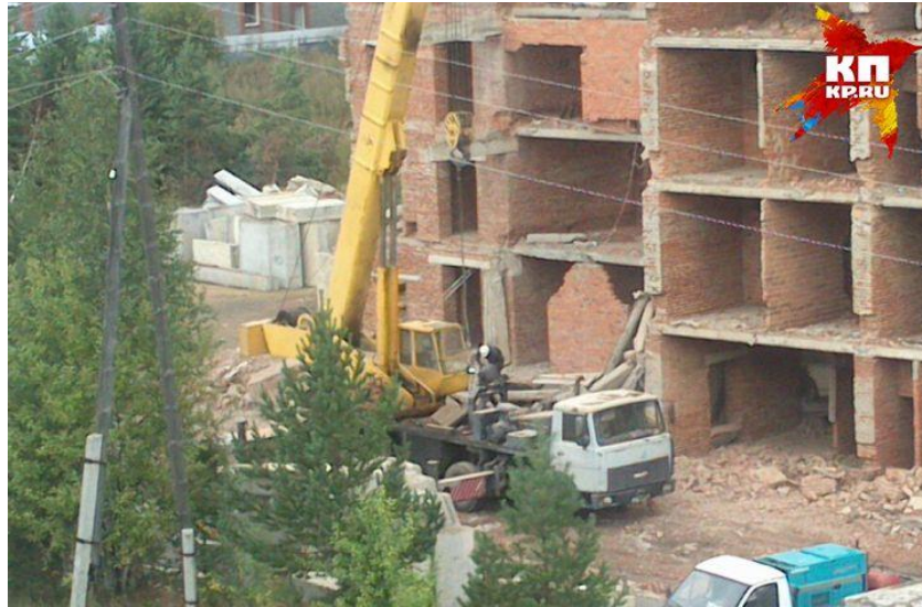
Fig. 3.7. The destruction building during construction, Ural, Russia, 2016
