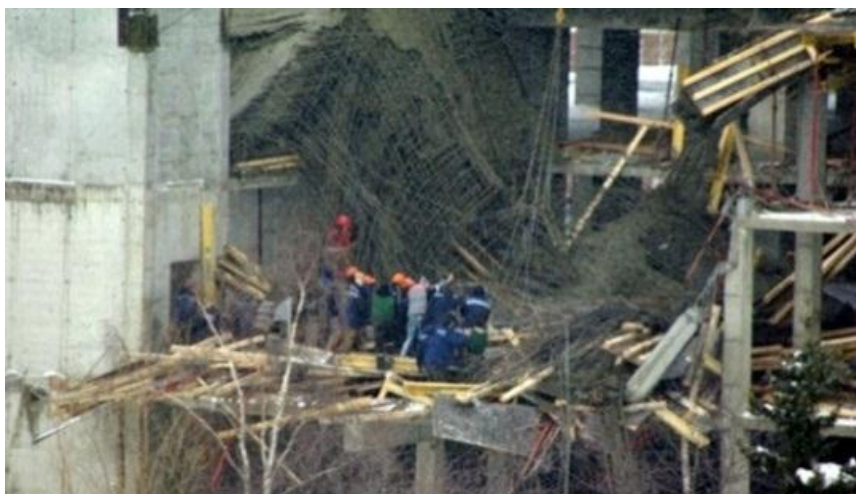
Fig. 3.5. Building collapse, Surgut, Russia, 2014
