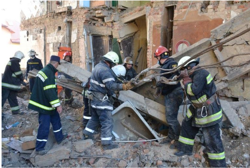
Fig. 3.10. Building collapse, Drobich, Ukraine, 2019
