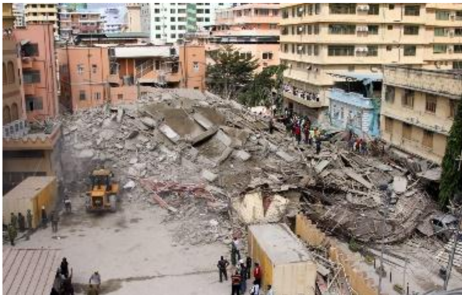
Fig. 3.3. Collapse of unfinished building, Dar es Salaam, Tanzania, 2013
