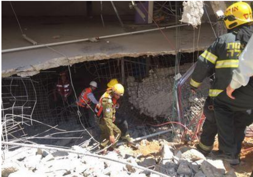
Fig. 3.6. Building collapse, Tel-Aviv, Israel, 2016
