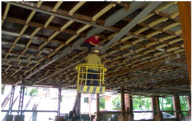
Fig.14: Fragment of overlap small-element sprengel truss with a span L = 18 m, Truskavets city, Lviv region, Ukraine
