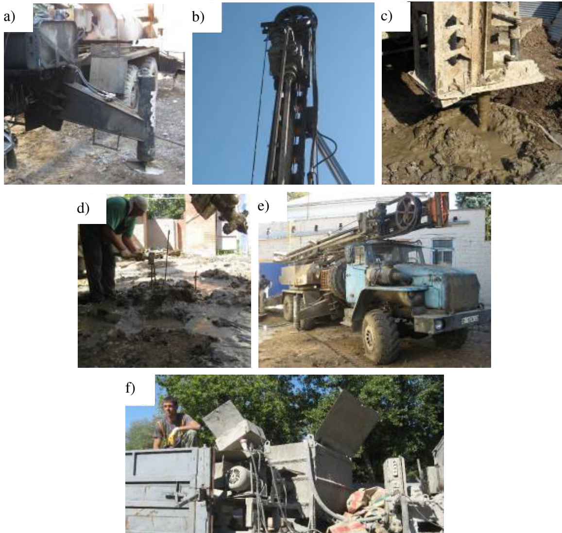
Picture 1 – Components of the process: a – supports deploying; b – adjustment of drilling tower; c – drilling; d – reinforcing bars placement into soil-cement; e – relocation of drilling device to next pile; f – supply with water-cement mixture
