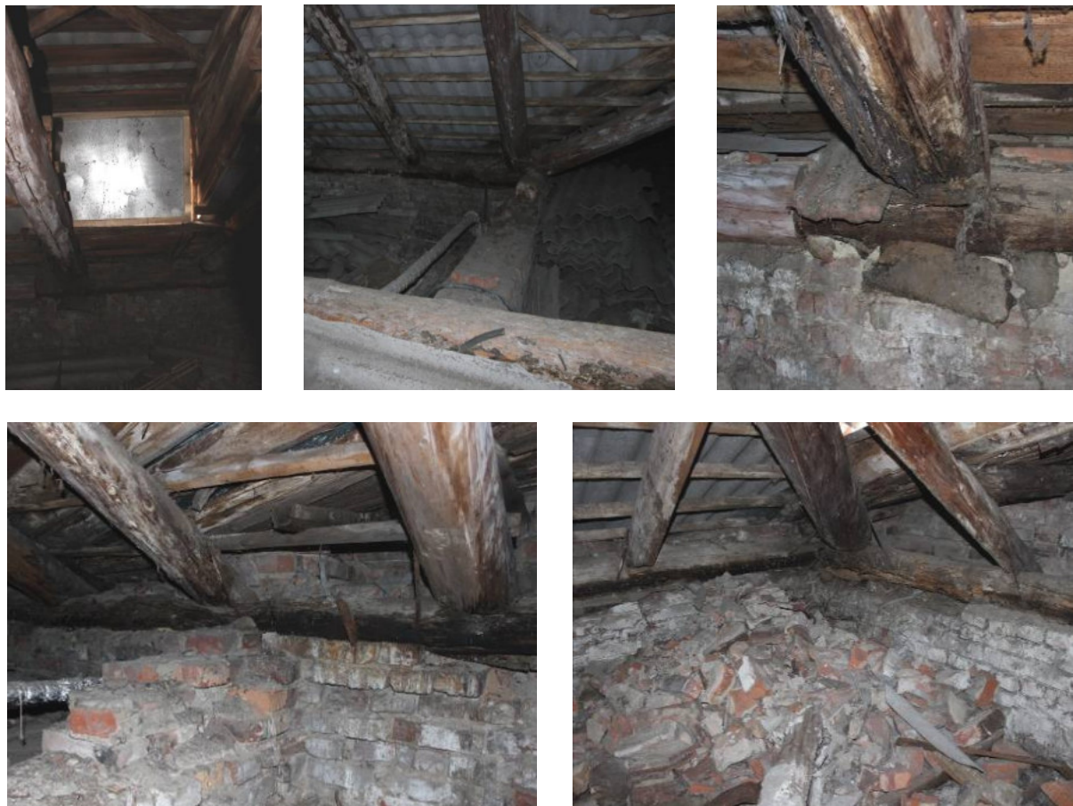
Figure 6 – Damage to wooden construction covering due to atmospheric and condensed moisture effect
