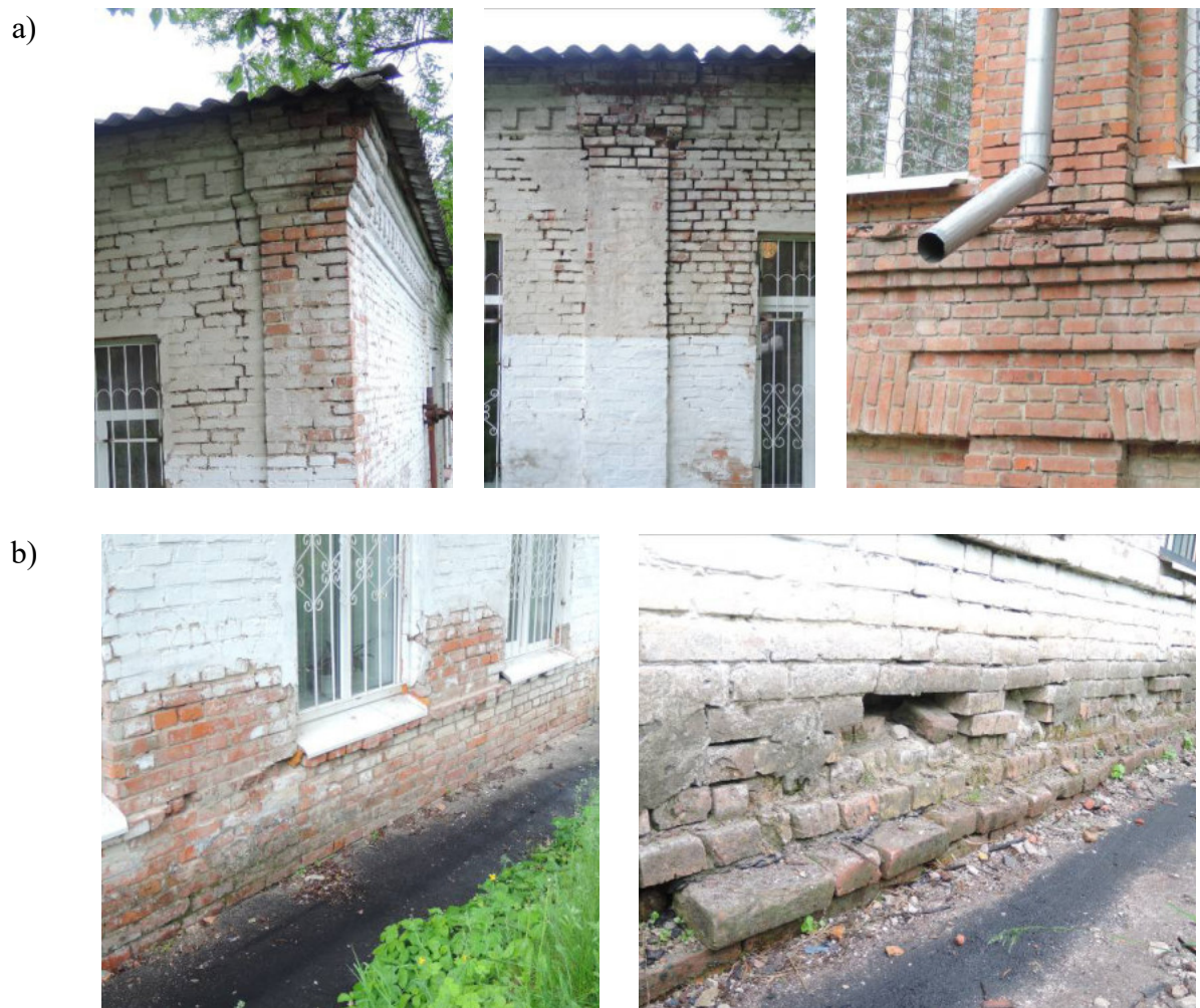
Figure 2 – Atmospheric moisture effects to brickwork of buildings enclosing structures: a) mortar weathering, frost destruction of the brickwork; b) water-saturation of the sole plate as a result of spraying water, fall of the brickwork fragments
