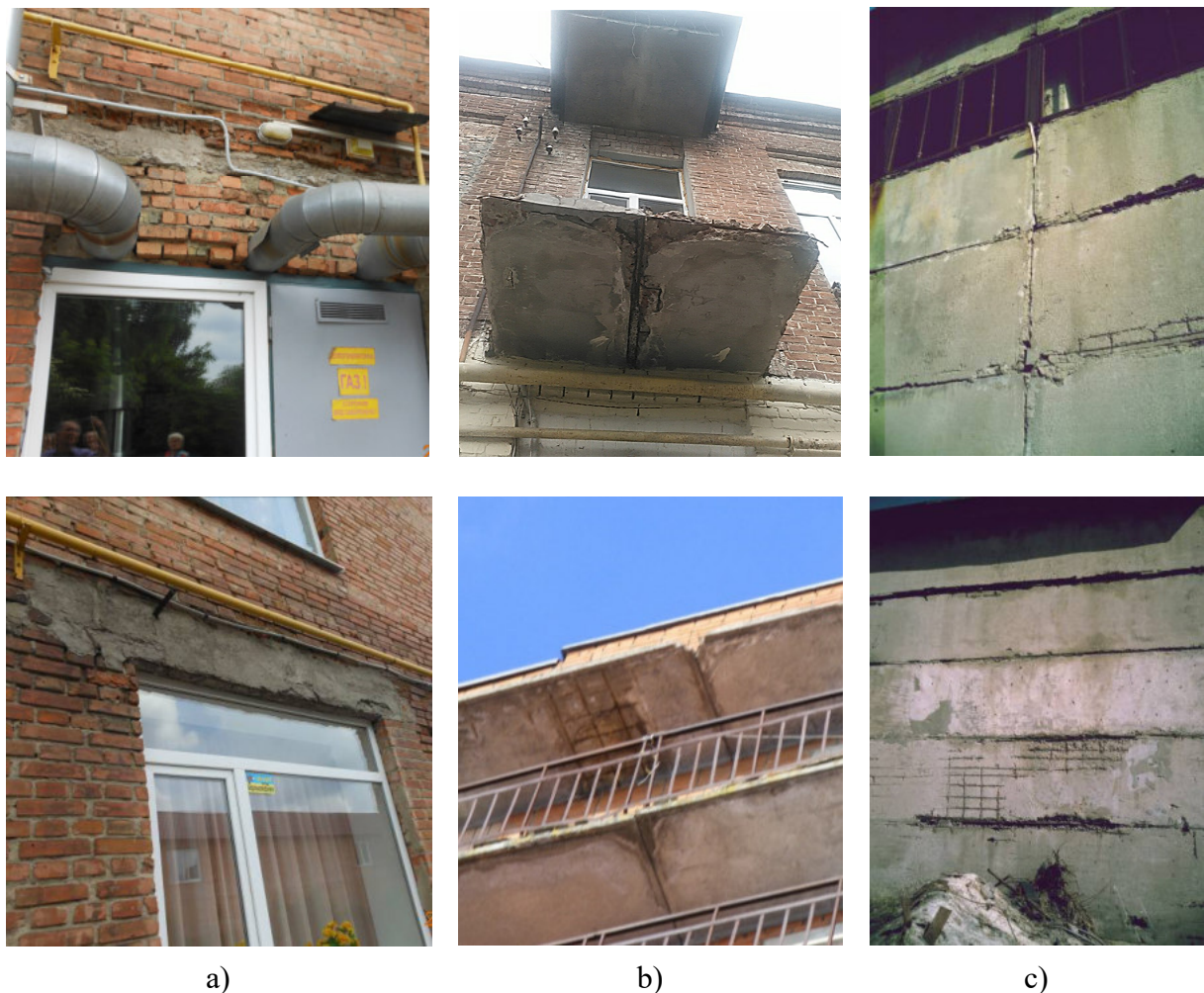
Figure 5 – Destruction of protective concrete layer of reinforced-concrete lintel (a), balcony plate (b), wall panel (c)
