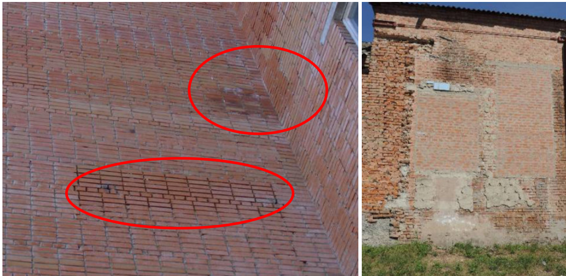
Figure 1 – Mortar ablation, brickwork frost destruction, the brickwork fragments fall, buildings enclosing structures brickwork local emergency sections due to the operational moisture impact
