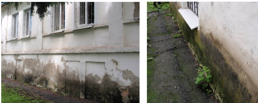
Figure 4. – Soil moisture effect as a result of destruction or lack of horizontal waterproofing, in case of banked up building sidewalks level above the horizontal waterproofing level
