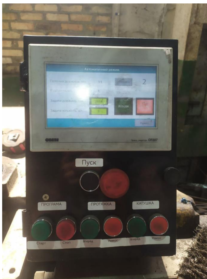
Figure 3.5 - Installed operator panel of the SP 307P, AQTECK
