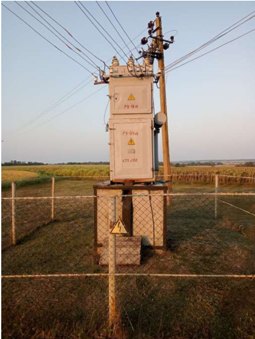
Figure 1.6 – Complete transformer substation
