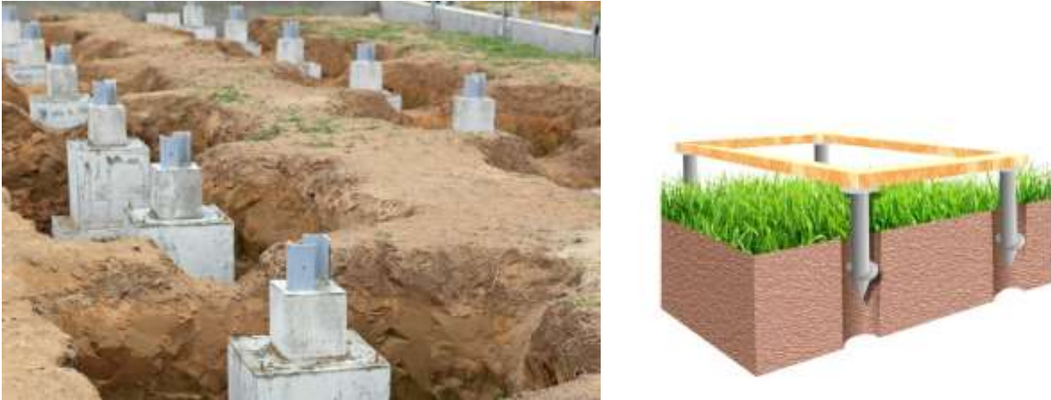
Figure 2 – Photo from performance of works on installation of the pile base, the scheme of a design of the pile base
