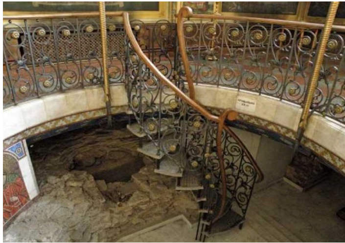
Fig. 8. The fragment of the monolithic reinforced concrete raft. [the archive of Ukrrestavratsiia Corporation]
