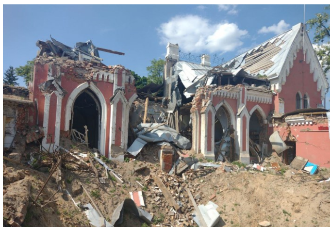
Fig. 1. The destroyed courtyard facade of Tamowski's mansion in Chernihiv
