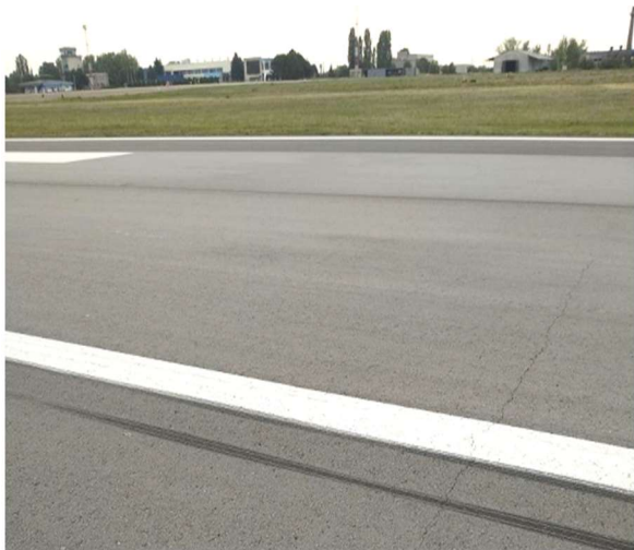
Figure 2 – Damage and defects of the "Mykolayiv International Airport" runway pavement
