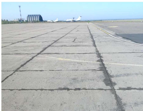
Figure 3 – Damage and defects of the "Mykolayiv International Airport" apron
