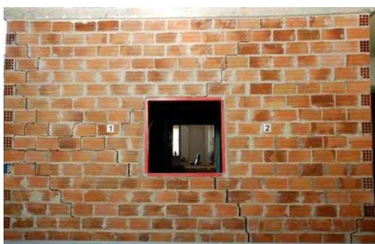
Figure 1 – The destruction nature of a fragment of masonry walls under seismic influences according to [3]
