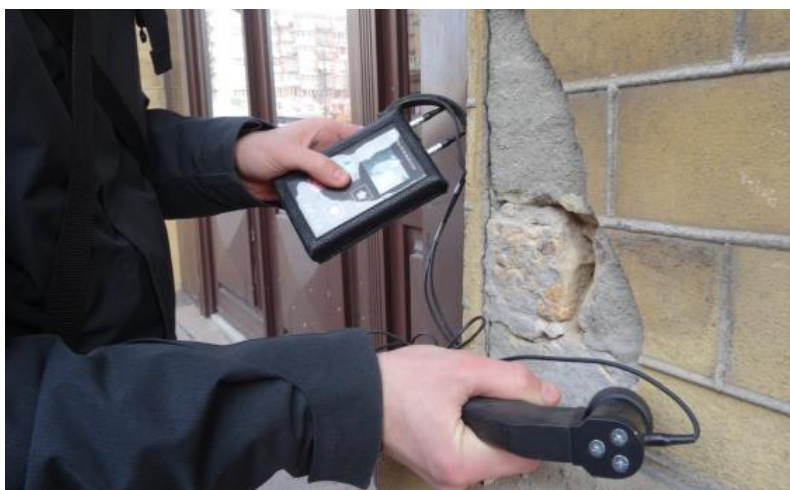
Fig. 4. The process of measuring the strength of stone facade structures. Photo by Oleksandr Molodid, 2021
