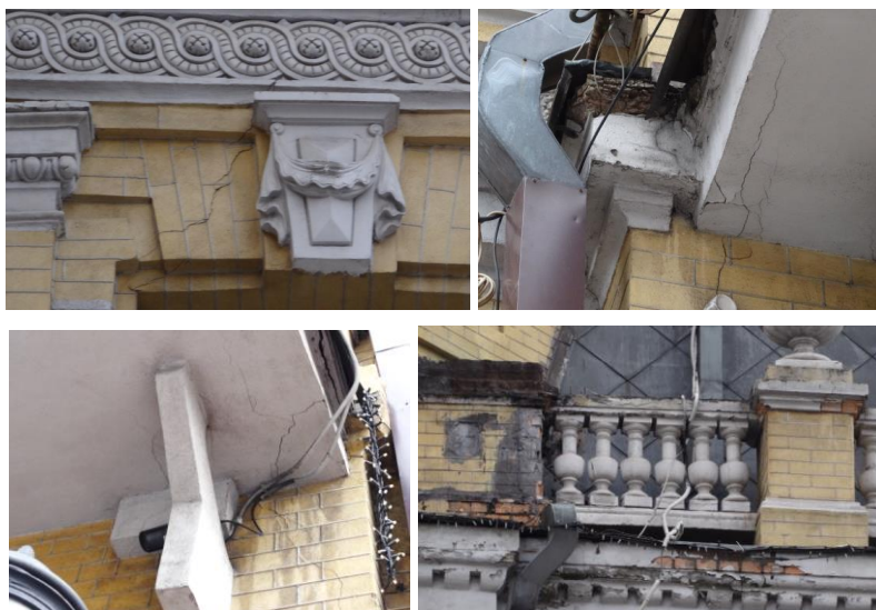
Fig. 6. Typical facade damages. Photos by Oleksandr Molodid, 2021
