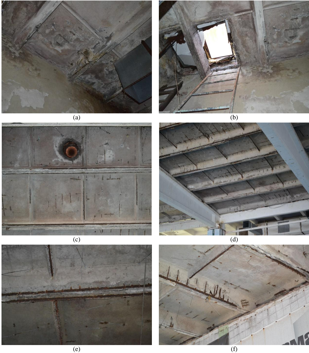
FIGURE 3. Characteristic damages of reinforced concrete structures of a covering during operation: white salt spots on the concrete surface (a), corrosion of concrete and reinforcement in places of design and non-design holes in reinforced concrete coating structures (b, c), peeling of the protective layer of concrete (d), corrosion of reinforcement, leading to the destruction of concrete, the loss of pieces of the protective layer of concrete ribs (e, f).
