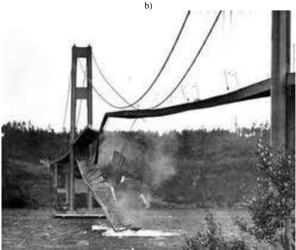
Fig. 3.2. Destruction of the Tacoma Bridge: a - the beginning of loosening; b - the nature of the bridge destruction
