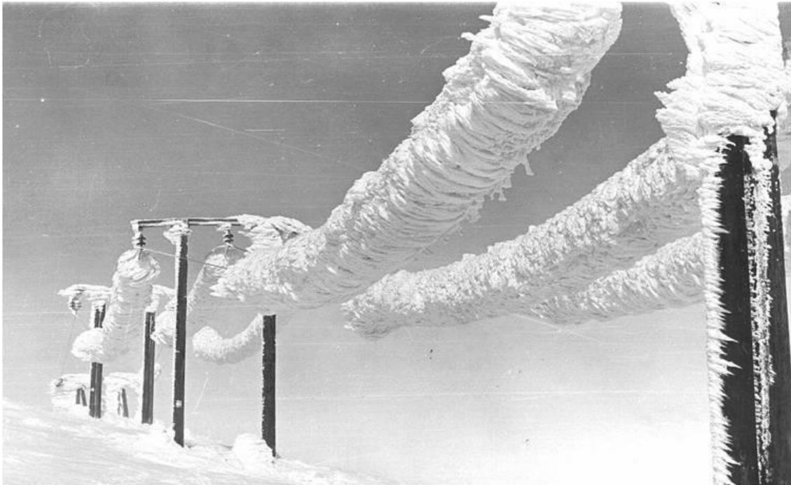
Fig. 15.1. Dangerous effects of ice: a - destruction of the OHL support from ice load; b - icing of electrical wires
