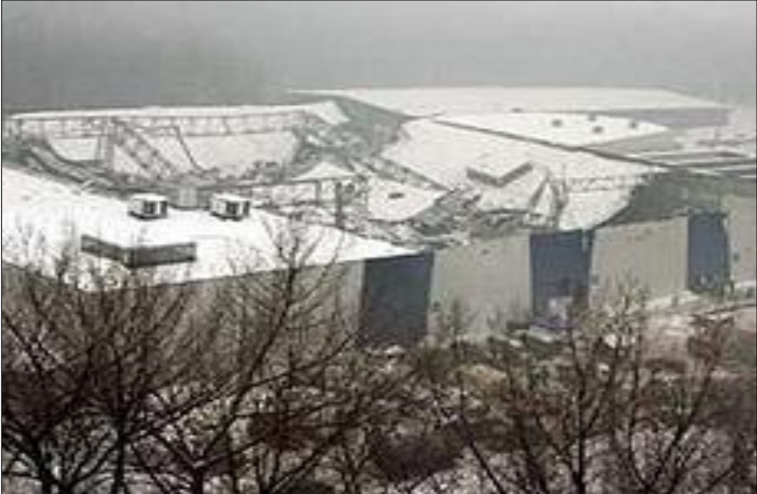
Fig. 9.4. Destruction of the pavement of the trade and exhibition pavilion (Katowice, Poland)
