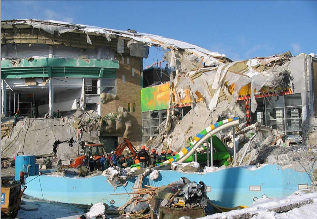
Fig. 9.3. Collapse of the sports complex (Bad Reichenwal, Germany)
