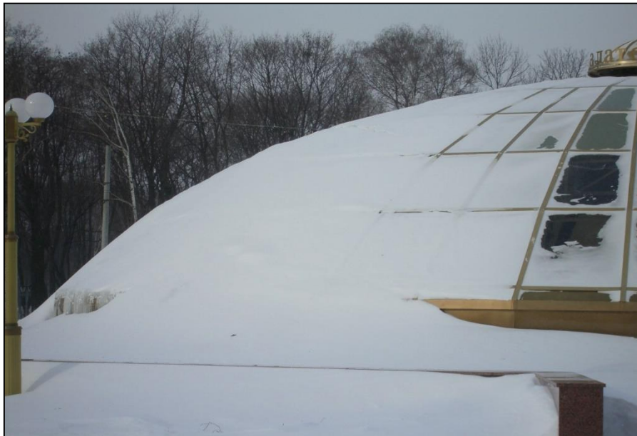
Fig. 10.9. Unbalanced snow load on the vaulted roof (underground passage "Golden City" in Poltava)
