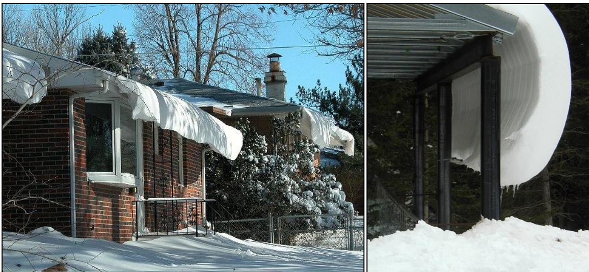
Fig. 10.12. Typical examples of snow hanging on roof eaves
